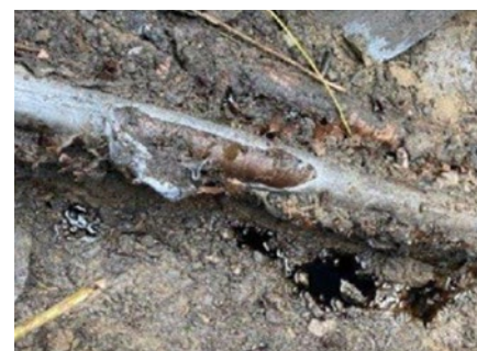
Damage to fluid-filled cable caused by house building contractor
