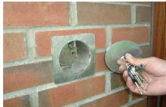
Figure 63: Example of Key Safe fitted in suitable location
